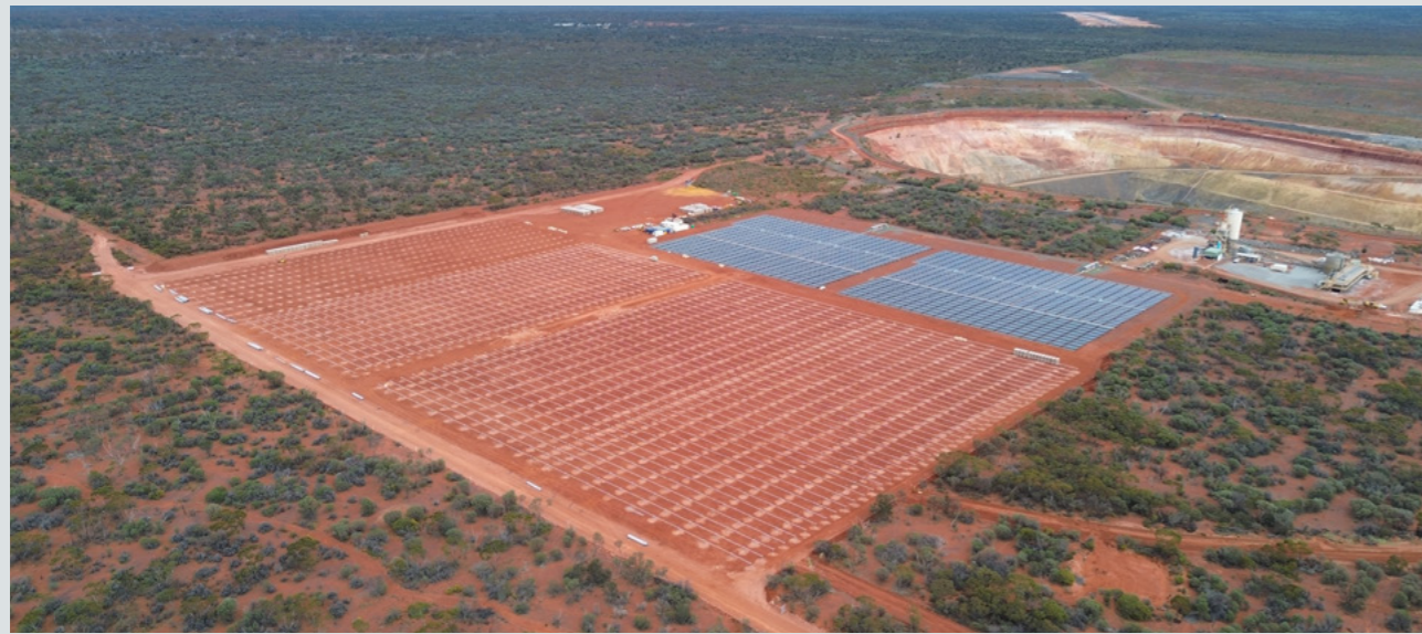
Figure 5 Clearing has been completed for the new 8MW solar plant at Carosue Dam Operations (existing solar farm adjacent)
