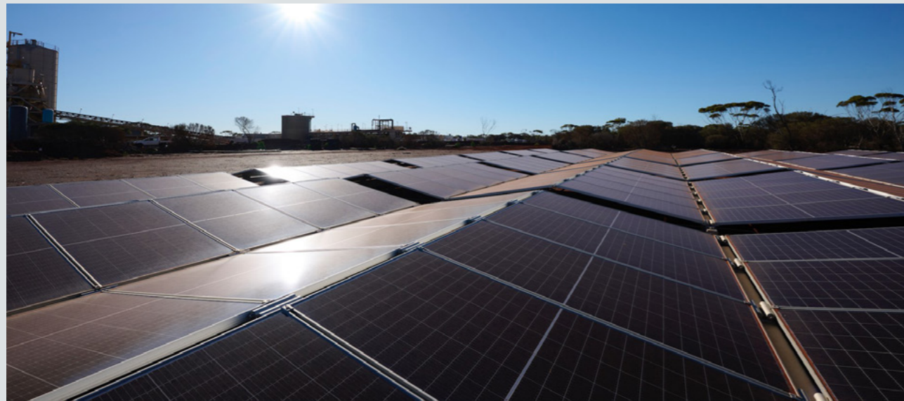
Figure 6 Existing solar array at Carosue Dam Operations
