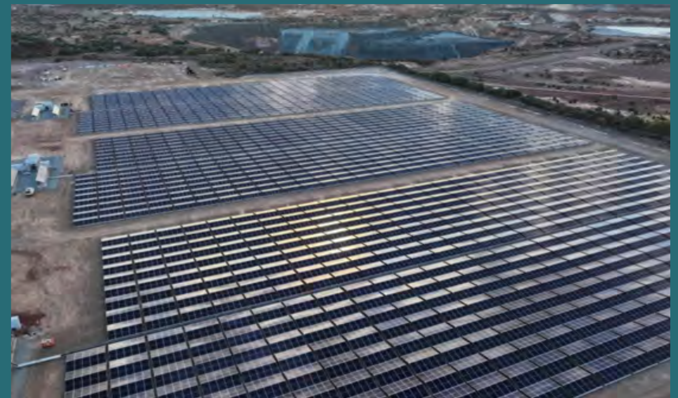
Figure 4 Completed solar farm at Jundee Operations
