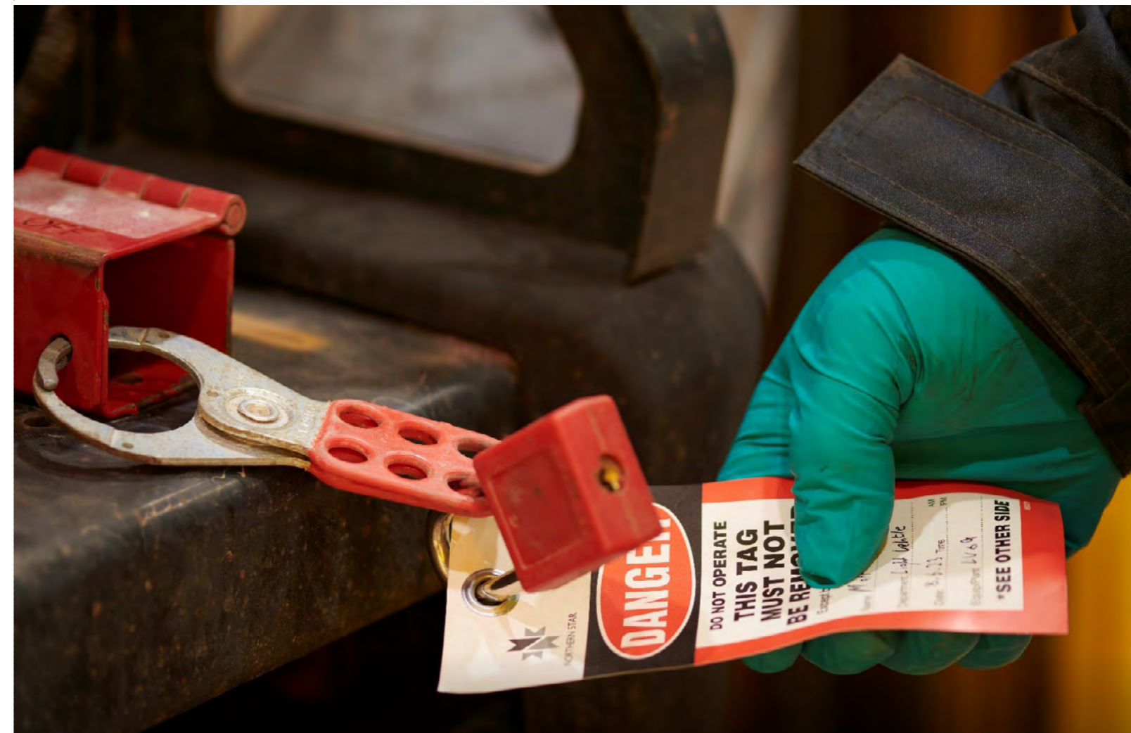
Isolation and lockout system in place at our LV Workshop, Jundee Operations, Yandal Production Centre, Western Australia
