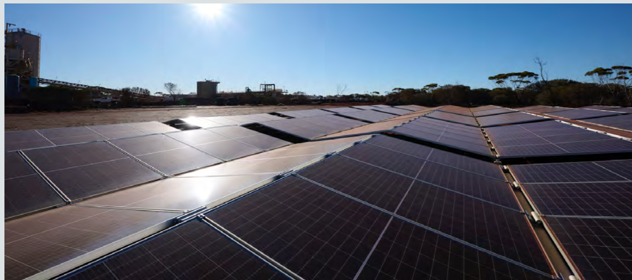
Figure 6 Existing solar array at Carosue Dam Operations
